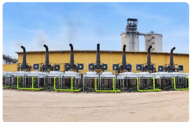
Industrial Power Station
