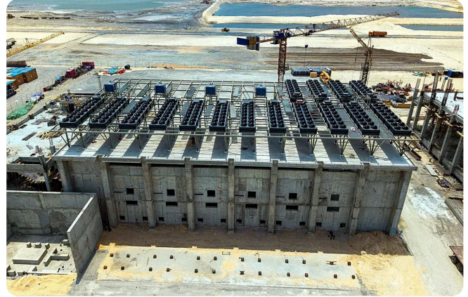
HFO Power Plant With TECS Radiators
